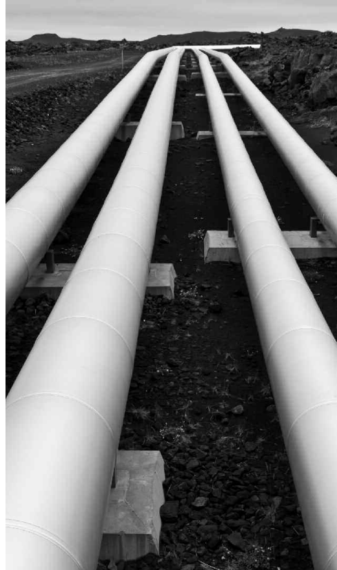
Geothermal power plant
