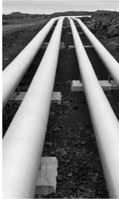
Geothermal power plant
