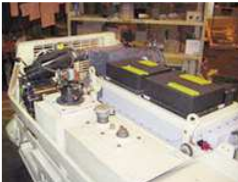
Closeup of a hybrid battery-diesel supply system in a Canadian loader by Mining Technologies International
