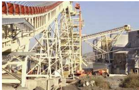
Conveyor system, after
