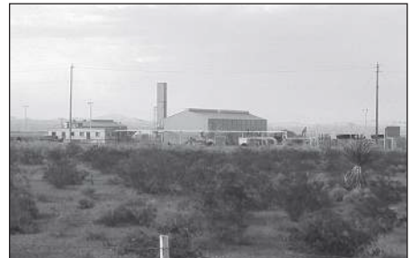
Natural Gas Compressor Station
